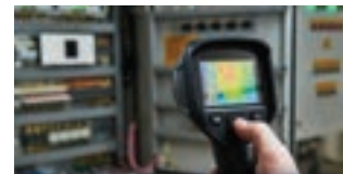
Thermography of Panels & Electrical equipments
